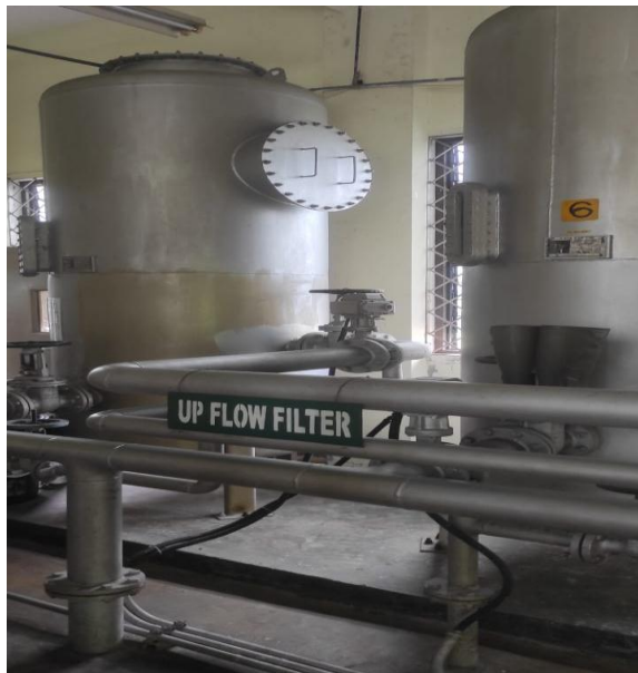
Sistem Up Flow Filter (Sistem Filterlisasi )
