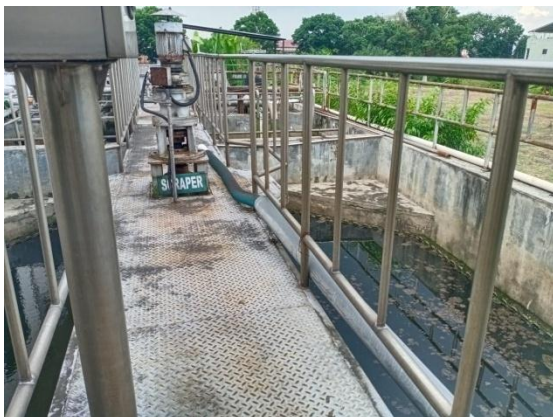
Bak Settling Bassin ( Bak Sedimentasi akhir )
