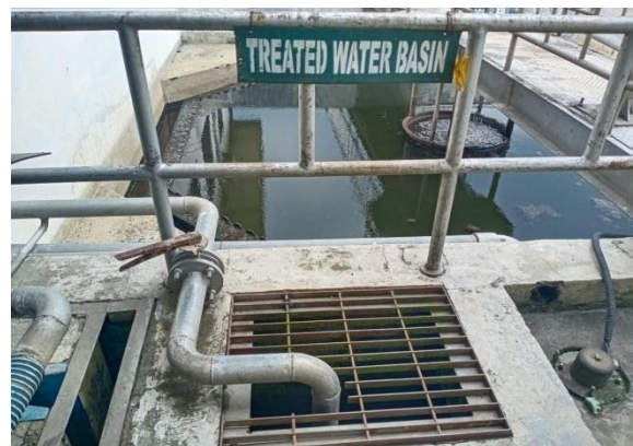
Bak Treated Water Basin dan Bak Desinfeksi
