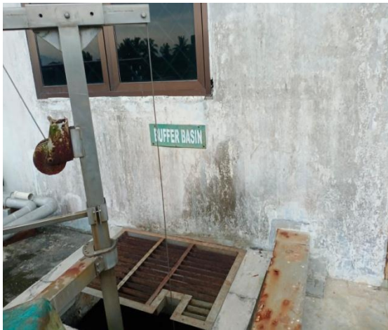
Buffer Bassin (Sedimentasi awal )
