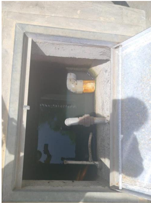
Gambar 9. Outlet (Treated water tank)
